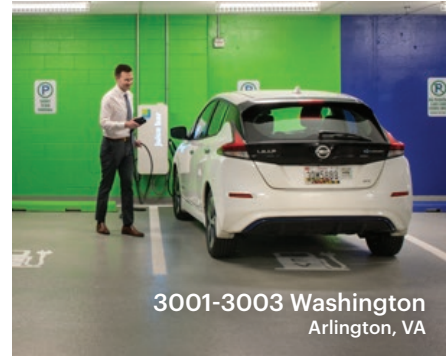
EV Charging Stations
